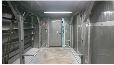
Area Blast Freezer
